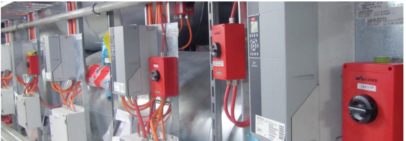
KEA Firerated safety switches installed at Keilaniemi metro station in Espoo, Finland
